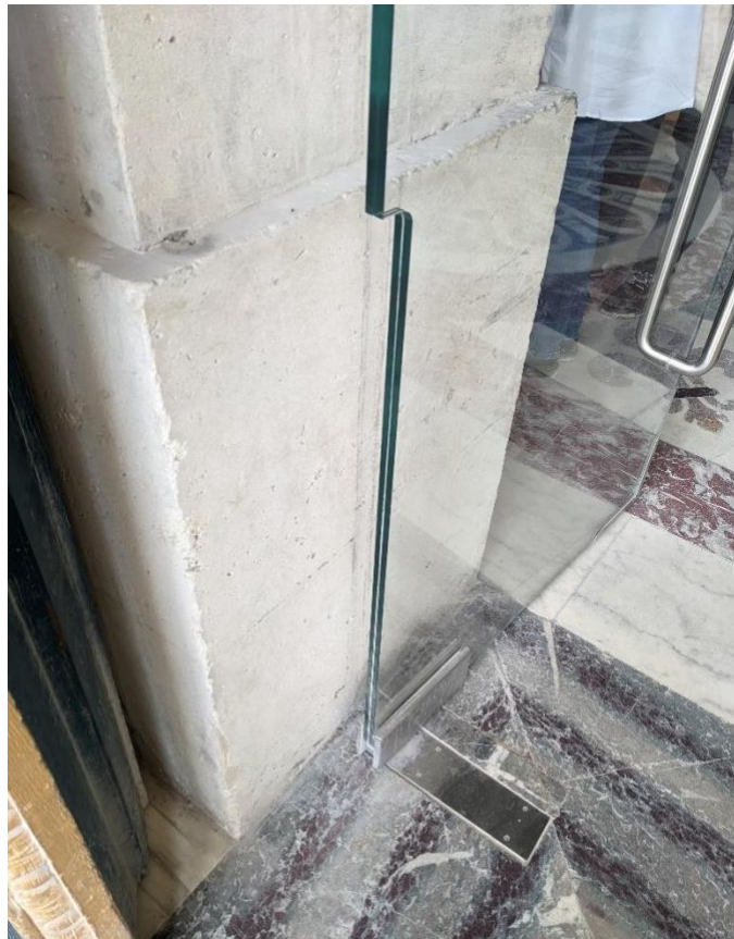
Figure 6: Detail at modern glass door with pivot hinge hardware at existing masonry opening.
