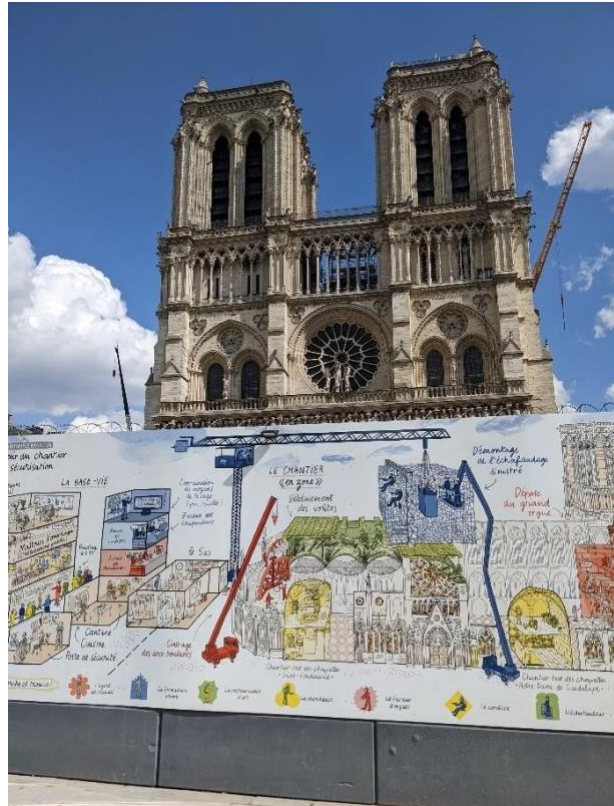
Figure 76: Notre Dame Cathedral under renovation; construction barriers contain great illustrations explaining the restoration work taking place.
