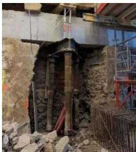
Figure 16: new concrete beam with steel support installed to make up for deteriorated existing foundations, found after excavation
