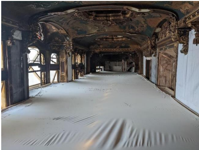
Figure 17: sheeting has been installed to protect future restoration area from new construction activities below.
