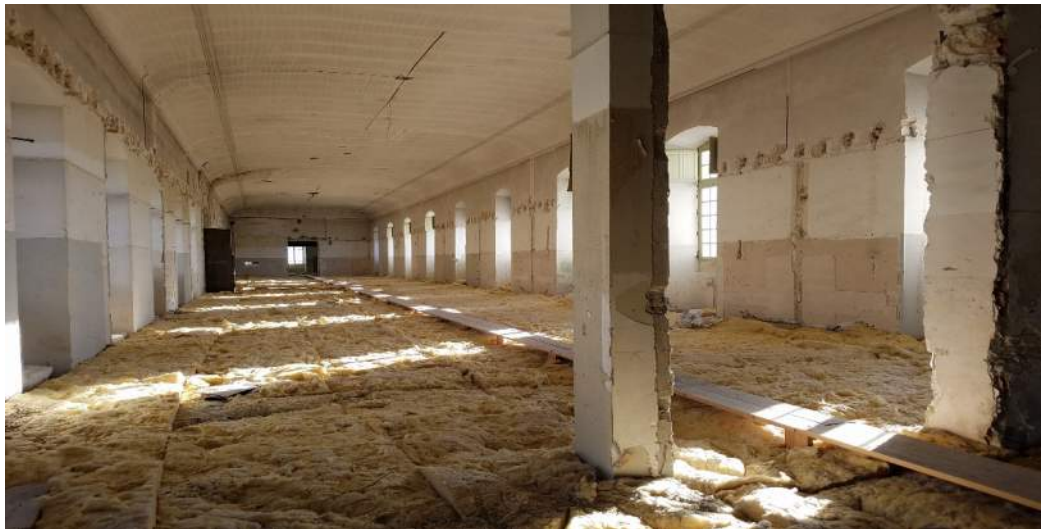
Fig. 5.6 L'inguimbertaine, la bibliothèque musée de Carpentras The manuscript room above occupied space (la bibliothèque musée de Carpentras). Wood planks were positioned to traverse the insulation like "acqua alta" in Venice Constance Lai. December 21, 2018.
